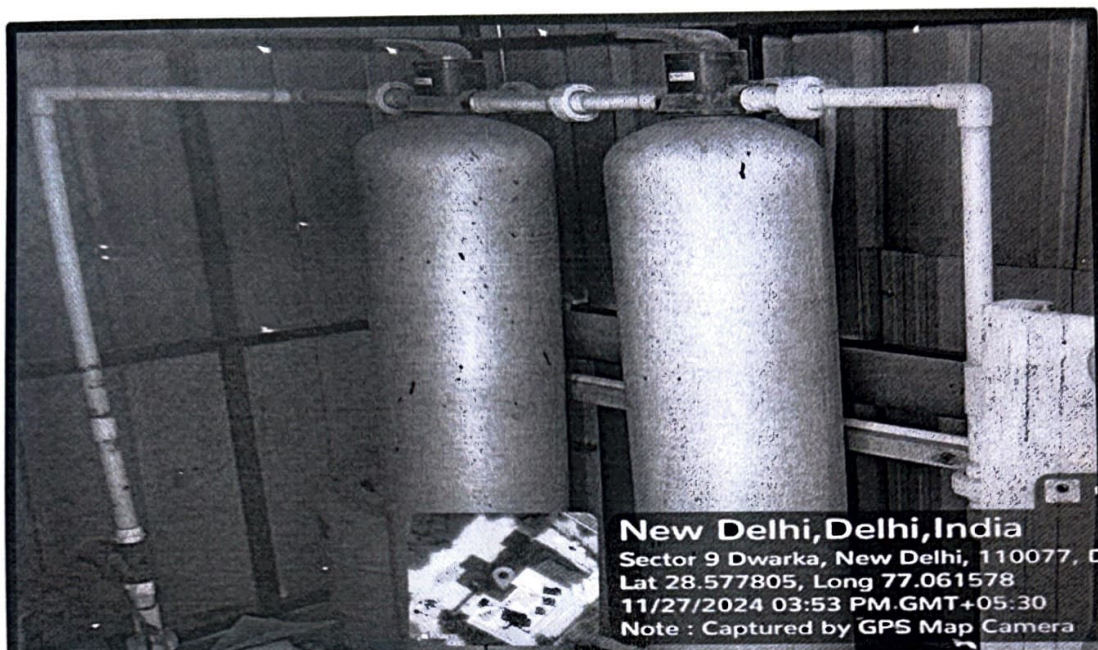
Innovative RO wastewater recycling
